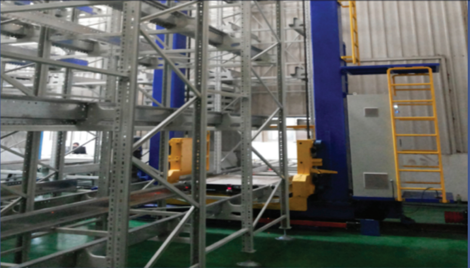
DOUBLE COLUMN STACKER CRANE + SHUTTLE CAR, AUTOMATIC WAREHOUSE
