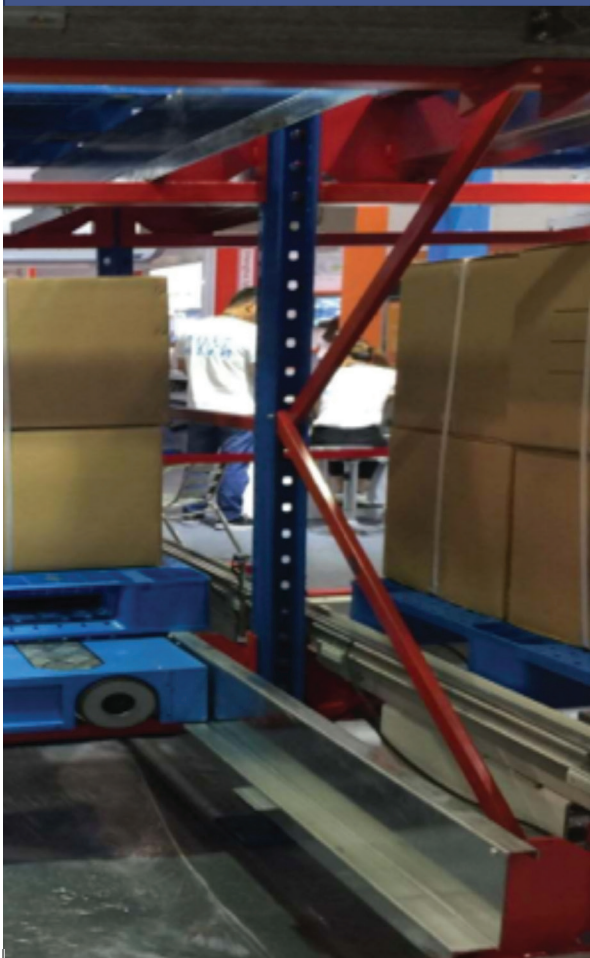
CRANE STACKER + FOUR-WAY SHUTTLE, AUTOMATIC WAREHOUSE
